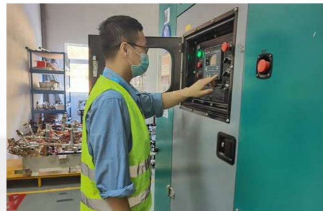
烟台 关闭辅助设备 YT Turn Off Auxiliary Equipment
