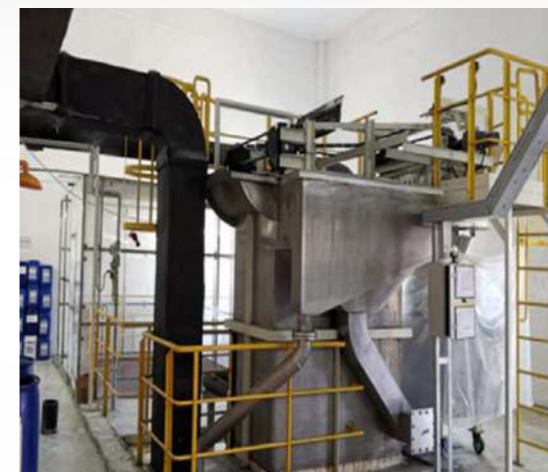
密封措施(刮渣池) Sealing measures (scraping pool)
